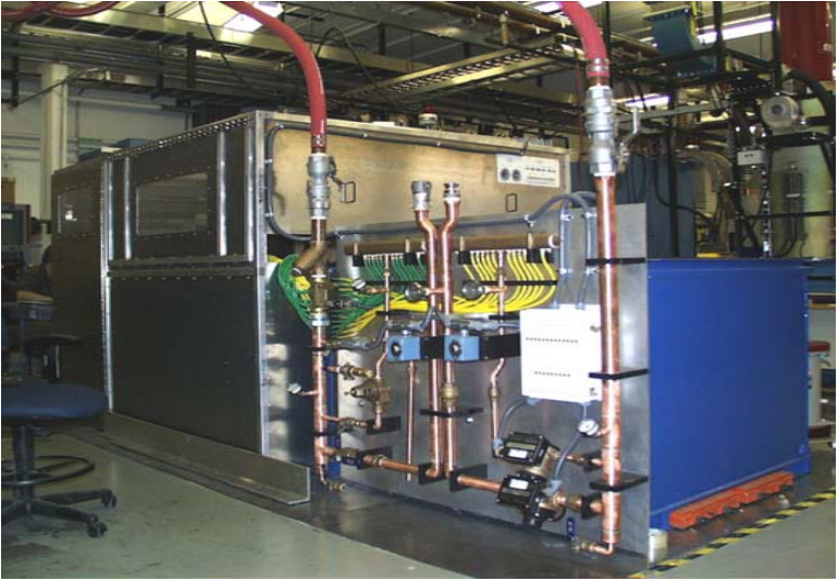
HIGH VOLTAGE CONVERTER MODULATOR
