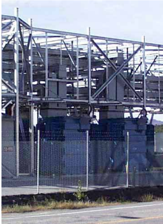
Typical H.V. Transformer
