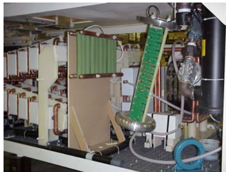
Oil Pump & Voltage Divider
