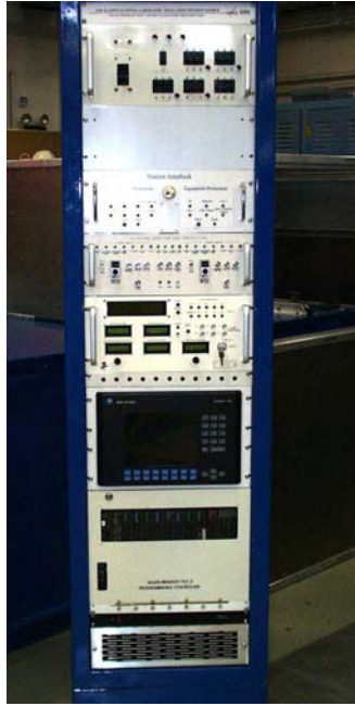
EQUIPMENT CONTROL RACK
