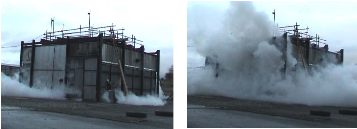
Figure 8. External view of rig during cold discharge test
