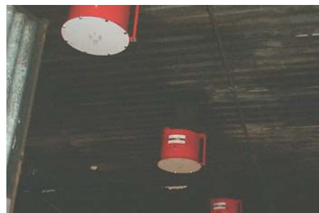
Figure 7. 11 kg units mounted on ceiling
