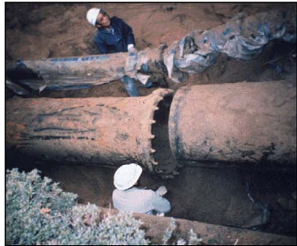
Figure 9-11. Joint Separation in Ductile Iron Pipe due to Liquefaction during 1995 Kobe Earthquake (Courtesy of Kobe Water Department)
