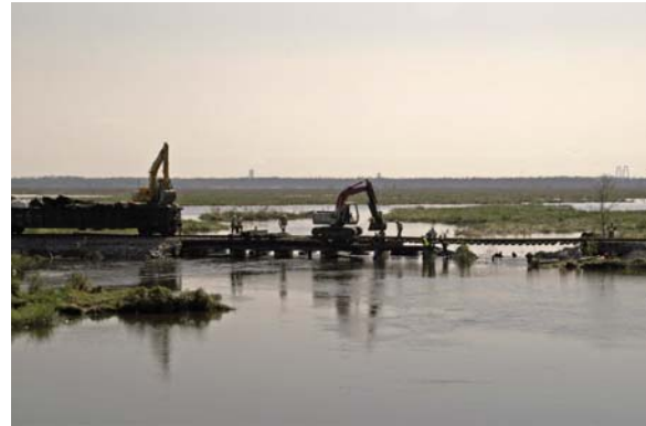
Figure 6-4: A railroad bridge in New Orleans is washed out by flooding (Photo by Marvin Nauman)
