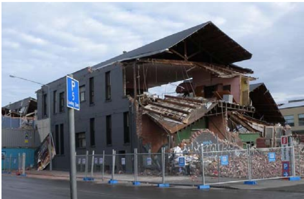
Figure 5-1: Failure of unreinforced masonry wall during an earthquake event. (Photo courtesy of Degenkolb Engineers)
