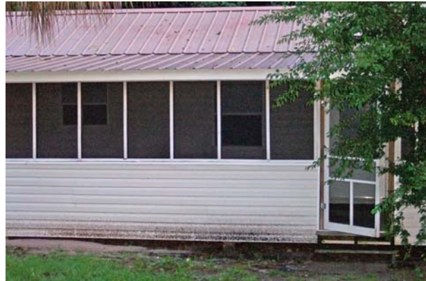
Figure 5-3: Floodwaters reached just under the first floor on this building (photo courtesy of AECOM)
