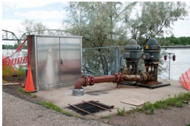
Figure 9-5. Bismarck, ND Pump Station Damaged by Flood Inundation from Adjacent Missouri River (Courtesy of FEMA)
