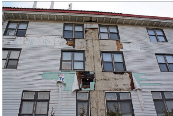
Figure 5-7: Siding loss and minor envelope damage on low-rise building from a wind event. (photo courtesy of FEMA) [getting a better quality version]
