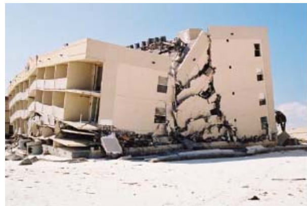
Figure 5-12: Collapse of 5-story building due to undermining (from flooding) of shallow foundation (courtesy of FEMA)
