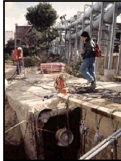
Figure 9-13. Higashinda WWTP Channel Offset by Liquefaction in 1995 Kobe Earthquake (Courtesy of Donald Ballantyne)
