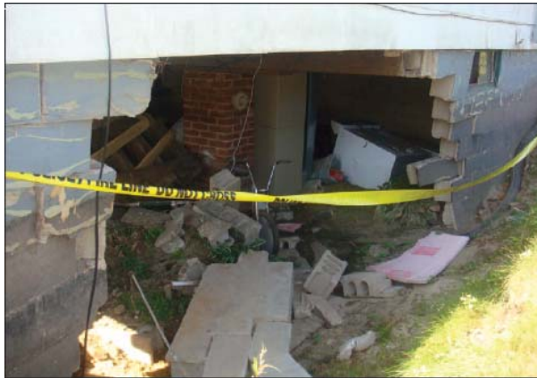
Figure 5-10: Foundation wall collapse due to hydrostatic pressure from floodwaters (courtesy of FEMA) [getting a better quality version]
