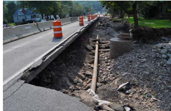
Figure 6-1: Road undercutting in the aftermath of Hurricane Irene (FEMA, Photo by Elissa Jun, 2011)
