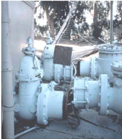
Figure 9-8. Tank Moved, Severing Connecting Pipe in 1994 Northridge Earthquake (Courtesy of Los Angeles Department of Water and Power)
