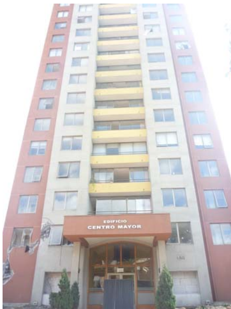
Figure 5-8: Apartment building with damaged structural members that is globally stable. (courtesy of Degenkolb Engineers)
