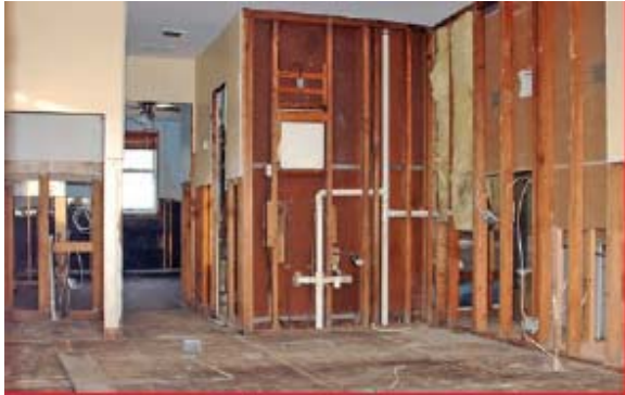
Figure 5-6: As a result of an estimated 3-4 feet of flooding, interior walls had to be replaced in this building, as well as an exterior door and window (photo courtesy of FEMA) [getting a better quality version]
