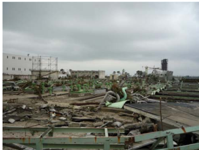
Figure 9-15. Sendai WWTP Equipment and Piping Damage from 2011 Earthquake (Courtesy of Donald Ballantyne)
