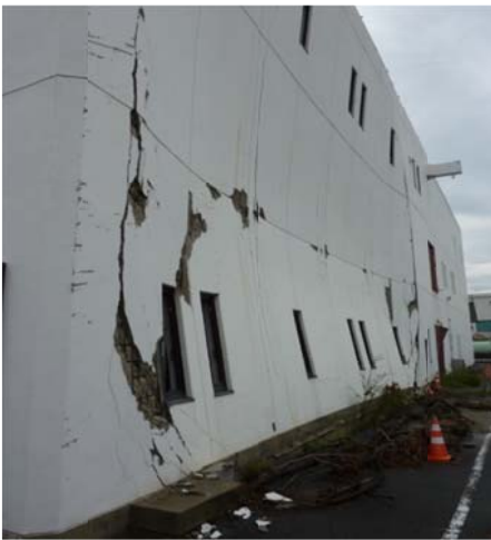
Figure 9-14. Sendai WWTP Effluent Pump Station Damaged by Tsunami in 2011 Tohoku Earthquake (Courtesy of Donald Ballantyne)
