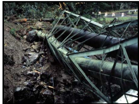
Figure 9-2. Water Transmission Pipeline Bridge Damaged by Landslide (Courtesy of Portland Water Bureau)
