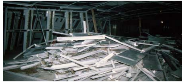
Figure 8-5. Light Fixture and Equipment Failure inside Central Office in Mexico City 1985 Earthquake (Alex Tang, OSSPAC 2013)
