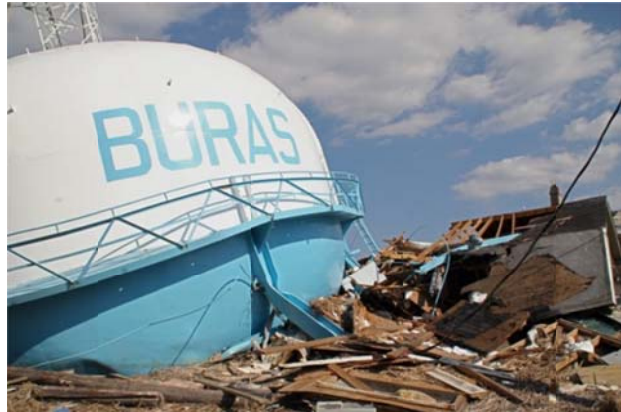
Figure 9-6. Collapsed Water Tank in Buras, LA near Hurricane Katrina Landfall Location (Courtesy of David Goldbloom- Helzner)
