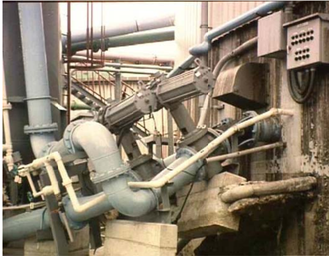
Figure 9-12. Non-Pile Supported Structures Failed Due to Liquefaction in 1995 Kobe Earthquake (Courtesy of Donald Ballantyne)
