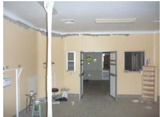
Figure 5-2: Non-structural damage to interior finishes following an earthquake event. (Photo Courtesy of Degenkolb Engineers)
