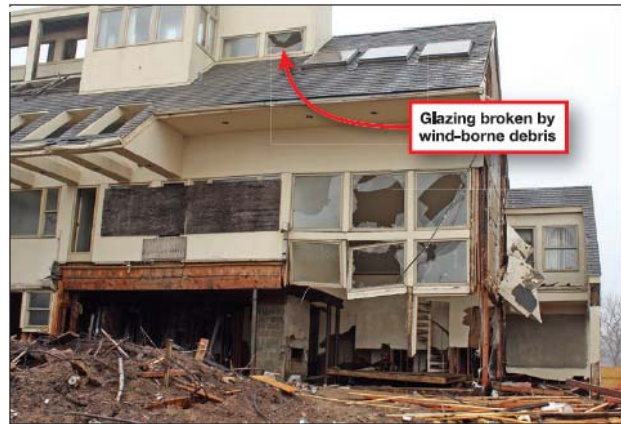
Figure 5-11: Wind and wind-borne debris resulted in considerable damage to glazing on this building (courtesy of FEMA) [getting a better quality version]
