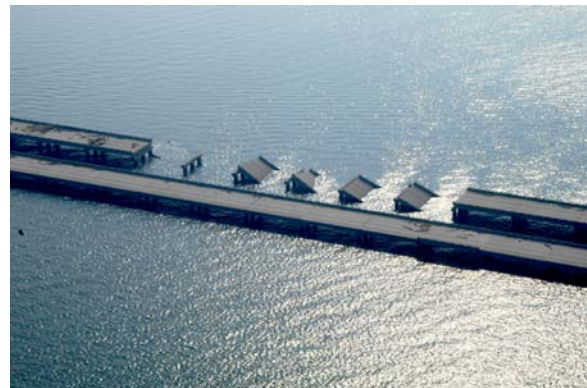
Figure 6-3: Bridge sections slid off their supports during Hurricane Katrina due to wave action (FEMA, 2005)
