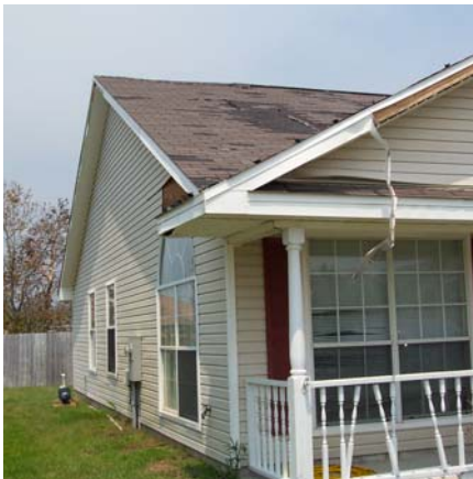
Figure 5-4: Damage to roof covering, vinyl siding and fascia as the result of wind (courtesy AECOM)
