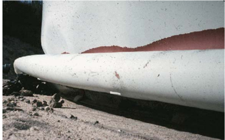
Figure 9-9. Steel Tank “Elephant’s Foot” Buckling in 1994 Northridge Earthquake (Courtesy of Donald Ballantyne)
