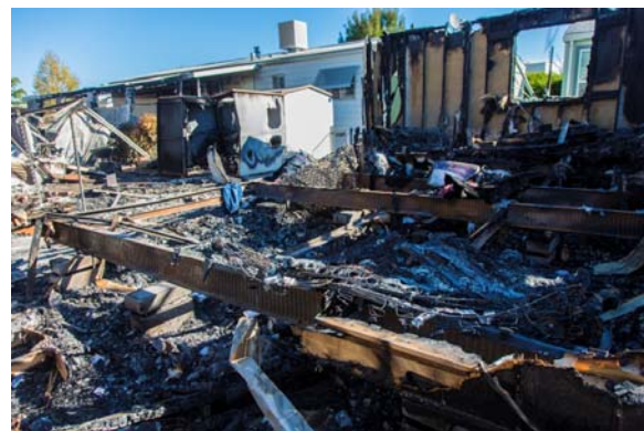
Figure 6-8: Fire damage from broken gas lines (Photographer: Christopher Mardorf, 2014)
