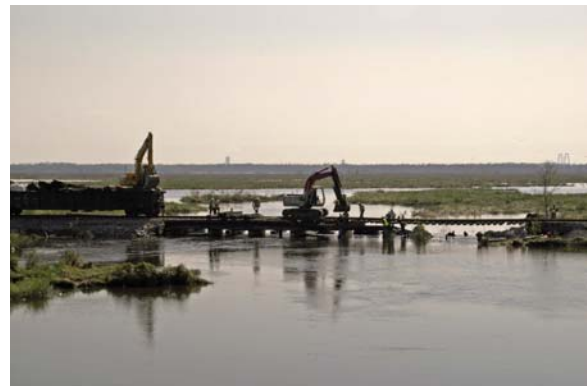
Figure 6-4: A railroad bridge in New Orleans is washed out by flooding.
