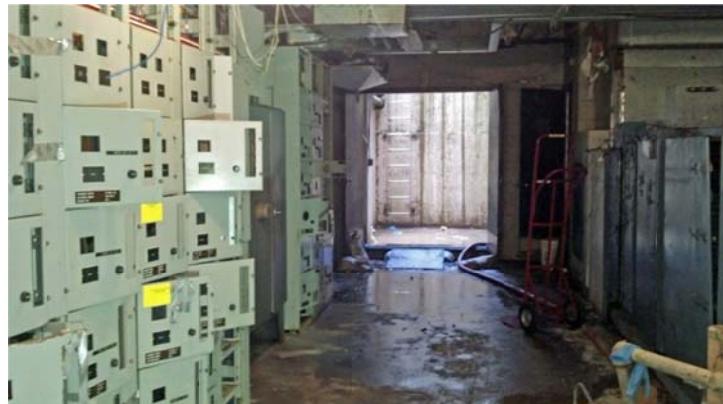
Figure 9-18: Subgrade Electric System Damaged By Floodwater at the Passaic Valley Sewerage Commission Wastewater Facility (FEMA, 2013)
