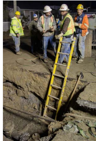
Figure 6-7: Natural gas crew shuts off gas after Hurricane Sandy (Photographer: Liz Roll, 2012)
