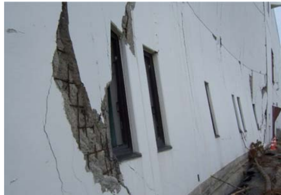
Figure 9-30: Structural Damage From Tsunami Wave and Debris Impact, Tohoku Earthquake, Japan, 2011 (Source: Tang & Edwards, 2014)
