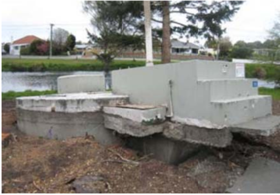
Figure 9-28: Pump Station Well Floated and Tilted Due To Liquefaction, Christchurch Earthquake, Christchurch, New Zealand, 2011 (Source: Eidinger & Tang, 2014)
