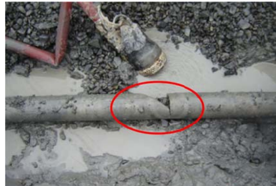
Figure 9-4: Water pipeline break, Christchurch earthquake, Christchurch, New Zealand, 2011 (Source: Eidinger & Tang, 2014)
