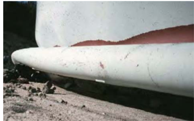
Figure 9-11: Steel Tank "Elephant's Foot" Buckling, Northridge Earthquake, California, 1994 (Source: Photo by Don Ballantyne)
