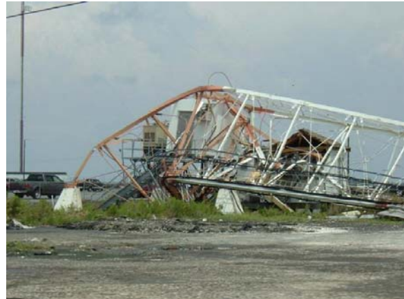
Figure 8-8. Tower Failed Due to Wind During Hurricane Katrina.
