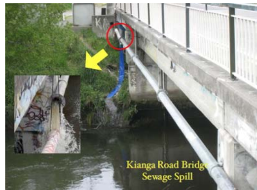
Figure 9-16: Sewer Pipeline Break Due To Bridge Support Settlement, Christchurch Earthquake, Christchurch, New Zealand, 2011 (Source: Eidinger & Tang, 2014)
