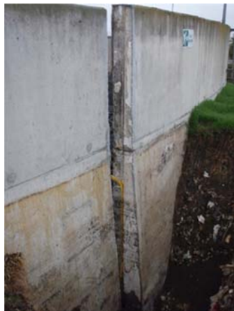
Figure 9-20: Process Tank Joint Offset Due To Permanent Ground Deformation, Maule Earthquake, Chile, 2010 (Source: Photo by Kent Yu)
