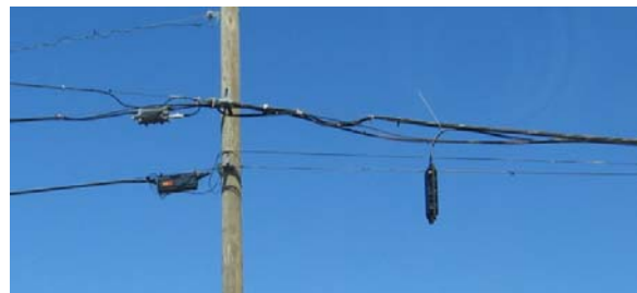
Figure 8-5. Failure of CATV cable due to the direct action of wind.
