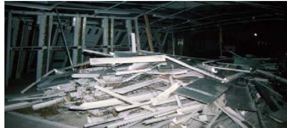
Figure 8-4. Light Fixture and Equipment Failure inside Central Office in Mexico City 1985 Earthquake (OSSPAC 2013)
