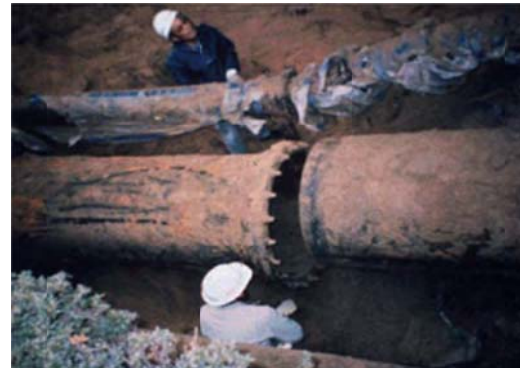
Figure 9-2: Pipeline Separated, Great Hyogoken-Nanbu Earthquake, Kobe, Japan, 1995 (Source: OSSPAC, 2013)
