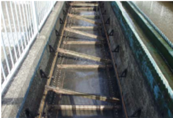
Figure 9-24: Damage To Chain-Driven Scraper, Tohoku Earthquake, Japan, 2011 (Source: Matsuhashi, et al., 2012 )
