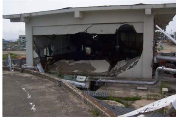
Figure 9-29: Structural Damage From Tsunami Wave and Debris Impact, Tohoku Earthquake, Japan, 2011 (Source: Tang & Edwards, 2014)
