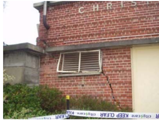
Figure 9-9: Pump Station Damage Due To Differential Settlement, Christchurch New Zealand Earthquake, 2011 (Source: Eidinger & Tang, 2014)
