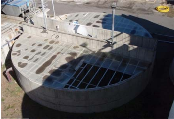
Figure 9-22: Process Tank Roof Damage Due To Sloshing, Maule Earthquake, Chile, 2010 (Source: Photo by Kent Yu)
