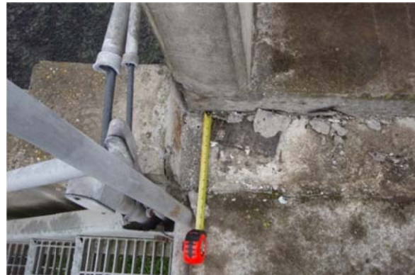
Figure 9-25: Damage To Electrical Conduit Due To Bridge Movement, Maule Earthquake, Chile, 2010 (Source: Photo by Kent Yu)
