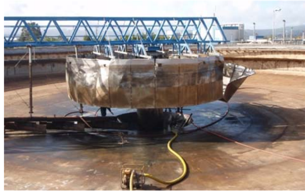
Figure 9-23: Clarifier Equipment Damage Due To Sloshing, Maule Earthquake, Chile, 2010 (Source: Photo by Kent Yu)
