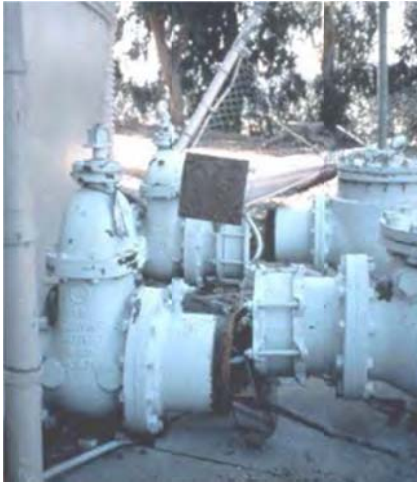
Figure 9-10: Tank Piping Separated, Northridge Earthquake, California, 1994 (Source: Schiff, 1997)
