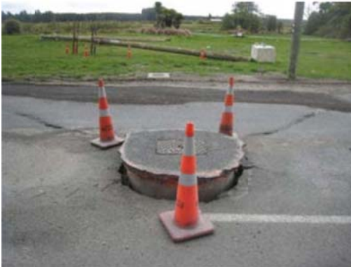
Figure 9-14: Manhole Floated due to Liquefaction, Christchurch Earthquake, Christchurch, New Zealand, 2011 (Source: Eidinger & Tang, 2014)
