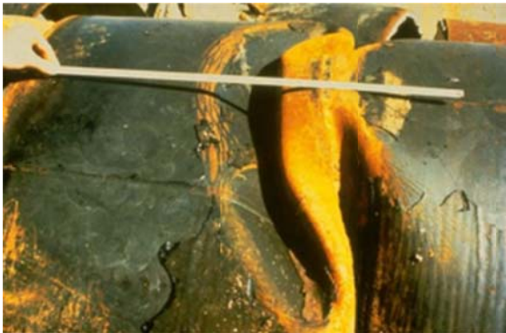
Figure 9-3: Welded Steel Pipe Compression Failure, San Fernando Earthquake, California, 1971 (Source: OSSPAC, 2013)
