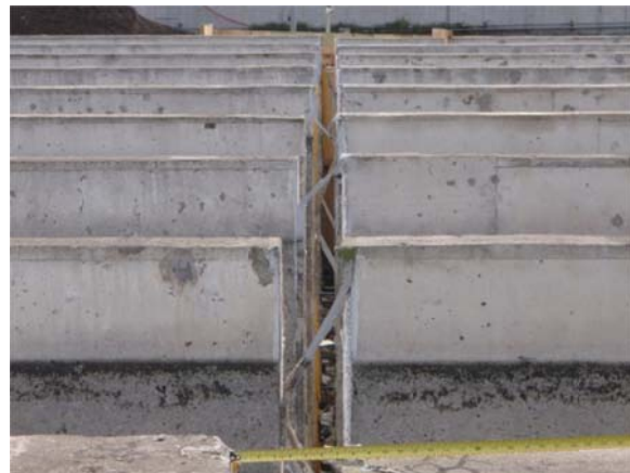
Figure 9-21: Chlorine Contact Tank Joint Separation Due To Permanent Ground Deformation, Maule Earthquake, Chile, 2010 (Source: Photo by Kent Yu)
