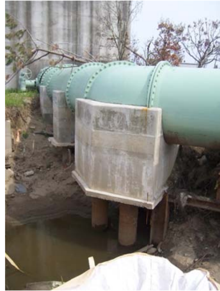
Figure 9-27: Eroded Pipe Support Foundation due to Tsunami Scour, Tohoku Earthquake, Japan, 2011 (Source: Tang & Edwards, 2014)
