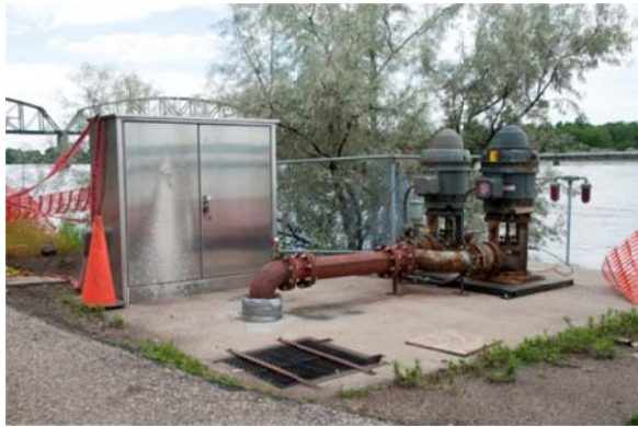
Figure 9-8: Bismarck, ND Pump Station Damaged By Flood Inundation From Adjacent Missouri River (Source: FEMA)
