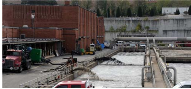
Figure 9-19: Floodwaters Are Pumped Out of Lower Levels of a WWTP In the Atlanta Area After Severe Storms Resulted In Significant Damage
