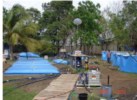
Figure 9-7: Temporary Water Treatment Plant, Haiti Port Au Prince Earthquake, 2010 (Source: Photo by Don Ballantyne)
