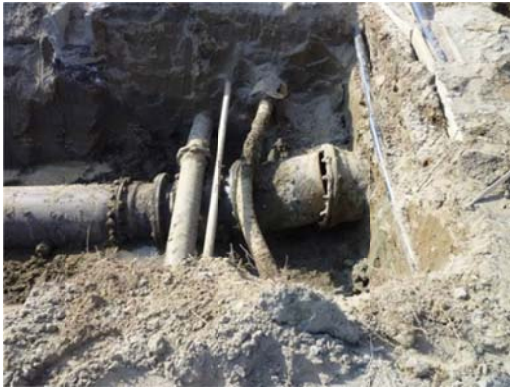
Figure 9-6: Pipeline Damage Due To Differential Settlement Between Ground and Pile Supported Building, Tohoku Earthquake, Japan, 2011 (Source: Tang & Edwards, 2014)
