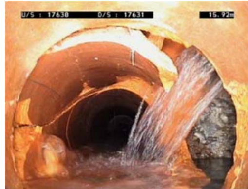
Figure 9-15: Sewer Pipeline Break, Christchurch Earthquake, Christchurch, New Zealand, 2011 (Source: Eidinger & Tang, 2014)
