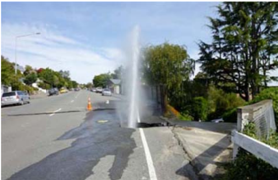
Figure 9-1: Water Pipeline Break, Christchurch Earthquake, Christchurch, New Zealand, 2011 (Source: Eidinger & Tang, 2014)
