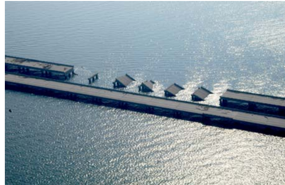
Figure 6-3: Bridge sections slid off their moorings during Hurricane Katrina due to wave action.
