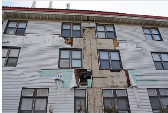
Figure 5-7: Siding loss and minor envelope damage on low-rise building from a wind event. (photo courtesy of FEMA) [getting a better quality version]
