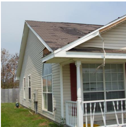
Figure 5-4: Damage to roof covering, vinyl siding and fascia as the result of wind (courtesy AECOM)
