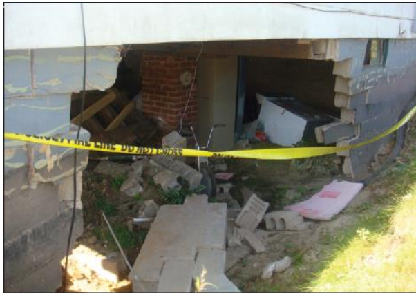
Figure 5-10: Foundation wall collapse due to hydrostatic pressure from floodwaters (courtesy of FEMA) [getting a better quality version]
