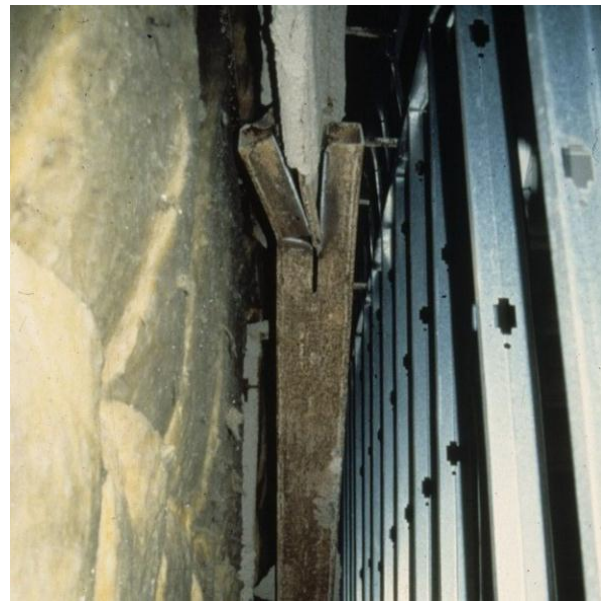
Figure 5-9: Fractured brace connection in a building damaged in an earthquake (courtesy of Degenkolb Engineers)
