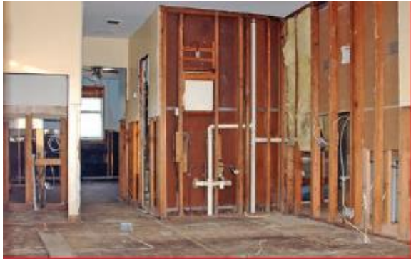
Figure 5-6: As a result of an estimated 3-4 feet of flooding, interior walls had to be replaced in this building as well as an exterior door and window (photo courtesy of FEMA) [getting a better quality version]
