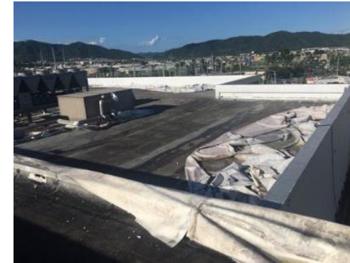
Damaged Roof Covering
