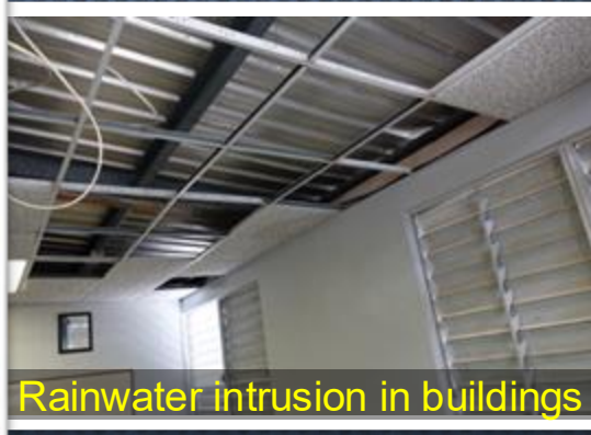
Building envelope damage
