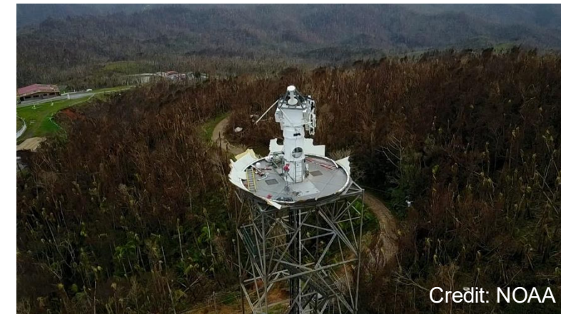
Failure of Doppler weather radar
