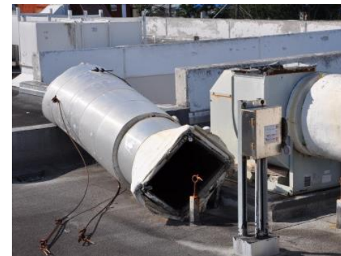
Damaged/Dislodged Rooftop Equipment
