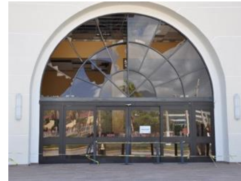
Windows with Broken Glass
