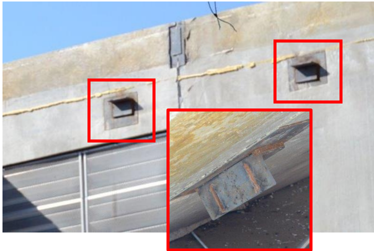
Weld Failure at Joist Seat
