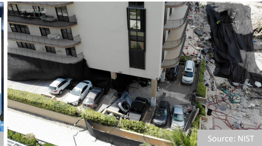
Eyewitness Accounts of Pool Deck Collapse
