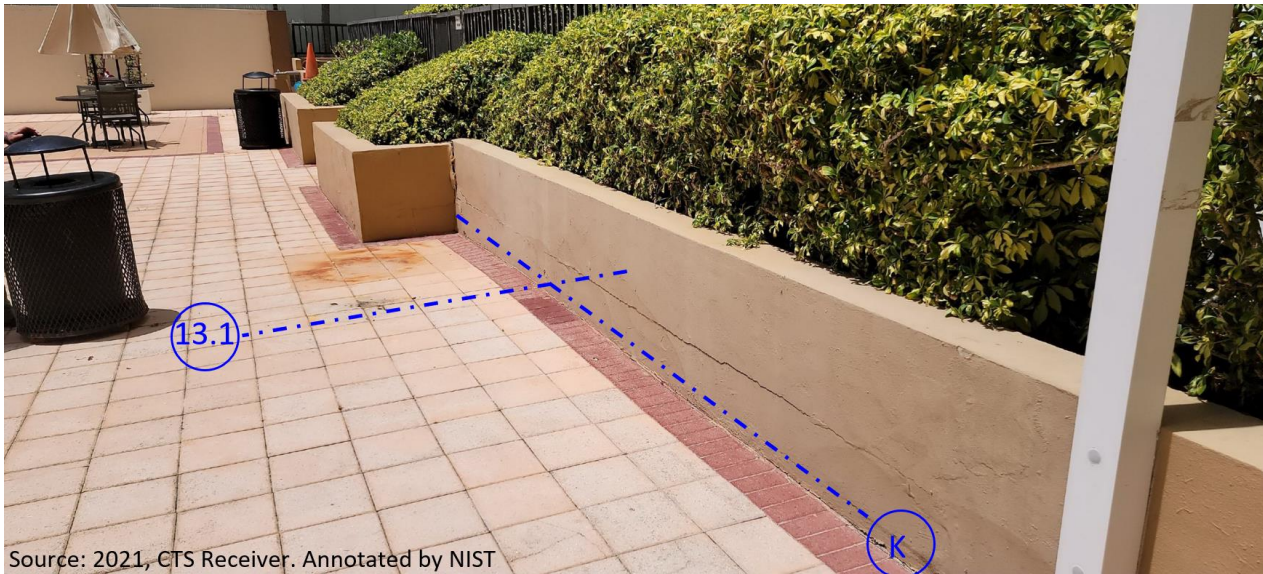
Damage to Pool Deck Planters Three Weeks Before the Collapse Indicated Severe Structural Distress
