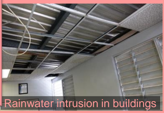
Building envelope damage
