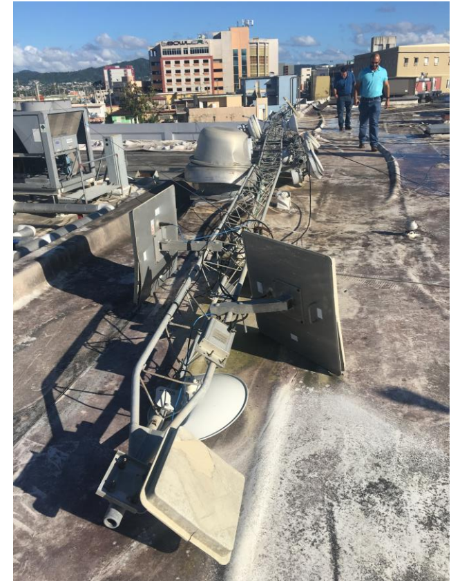
Collapsed Roof-Mounted Tower in Caguas
