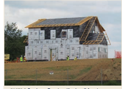
PHOTO 3 Overhang Framing. "Lookout" framing added over the top of the membrane. Rigid insulation is cut to fit into the "lookout" frame cavities and then covered with a continuous layer (or two) of insulation.
