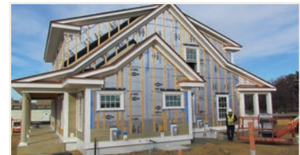
PHOTO 4 Continuous Insulation. The entire airtight assembly is insulated above grade with continuous insulation. In this case two layers of 2 in. (50.8 mm) foil faced polyisocyanurate. Could have been XPS or EPS or rockwool up to 8 in. (203 mm) thick.
