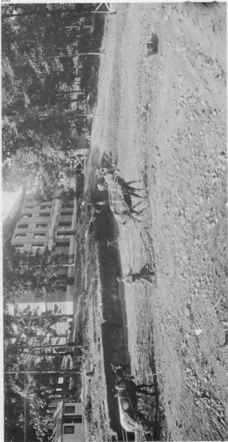
Mule teams leveling the ground for the new Chemistry building in the early fall of 1915. The rear of North building and the edge of the Low Temperature laboratory are in the background.
