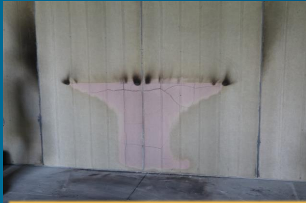
Cracking of cement board
