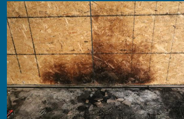
Significant thermal damage to OSB
