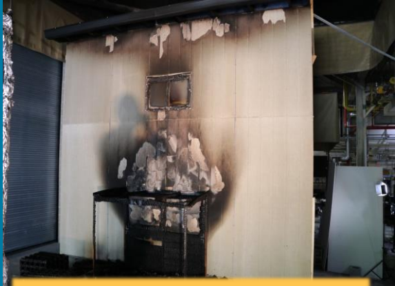
Significant spalling of cement board
