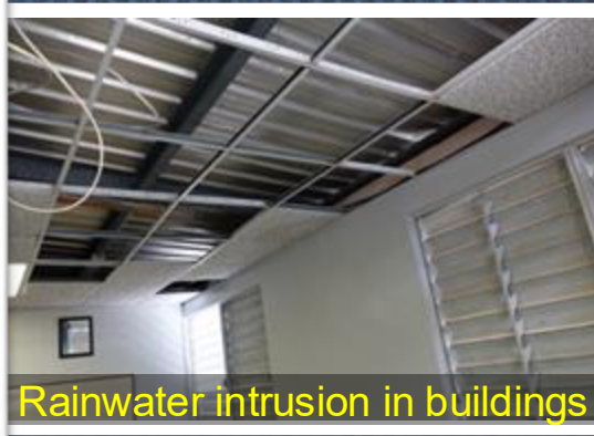
Building envelope damage
