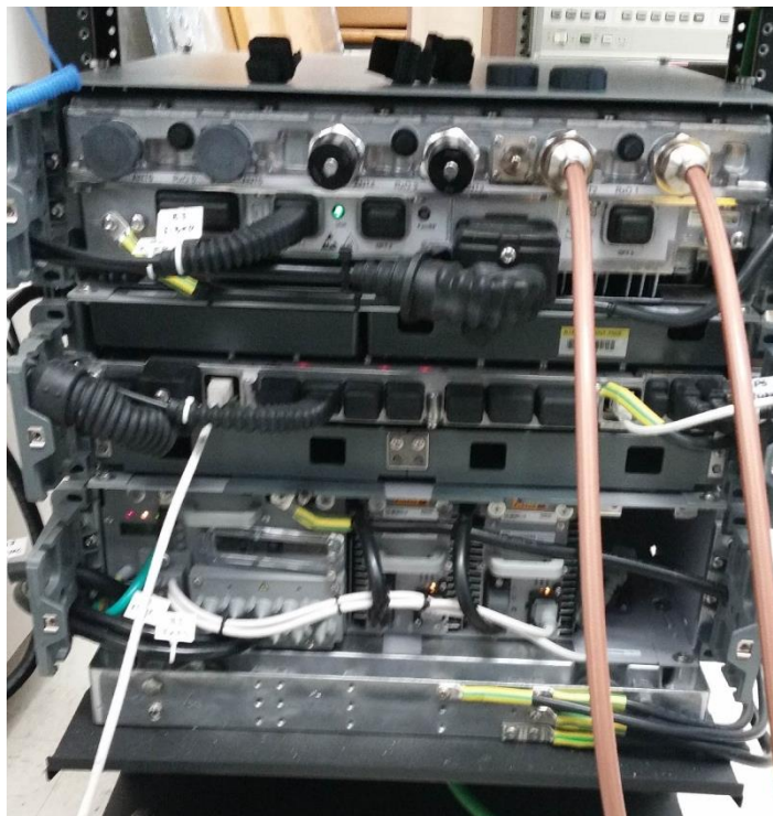
Figure A-9. The eNodeB hardware used in Phase I. The bottom of the three units is the power supply, the middle the CPU, and the top the remote radio head.
