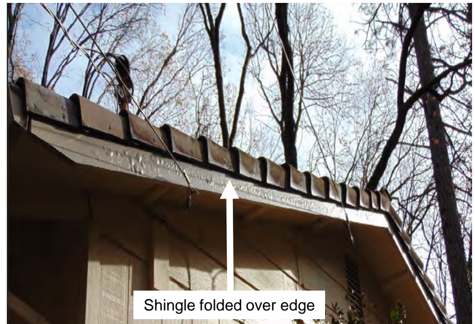
Item 8.3 & 9 No Gutters – Roof edge without gutters can leave combustible roof materials exposed.
