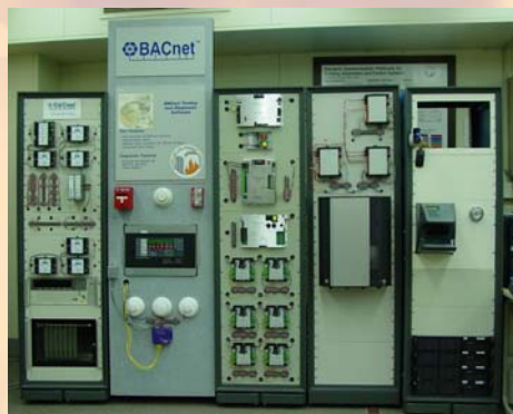
NIST Virtual Cybernetic Building Testbed Facility – Used to conduct research in automated fault detection and other aspects of integrated building control systems
