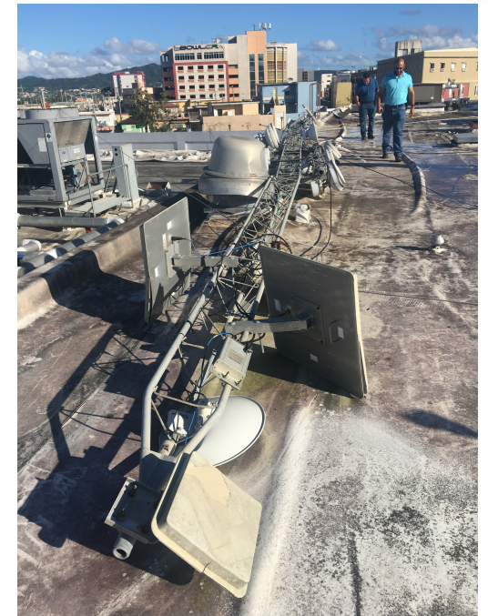
Collapsed Roof-Mounted Tower in Caguas
