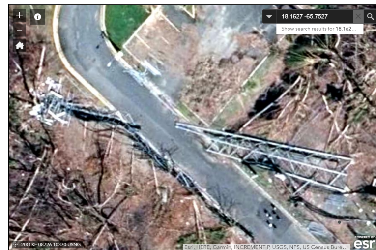
Collapsed Trussed Tower in Humacao
